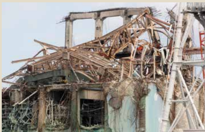
This damaged building at the Fukushima Daiichi nuclear power plant was photographed one year after the earthquake and tsunami.
