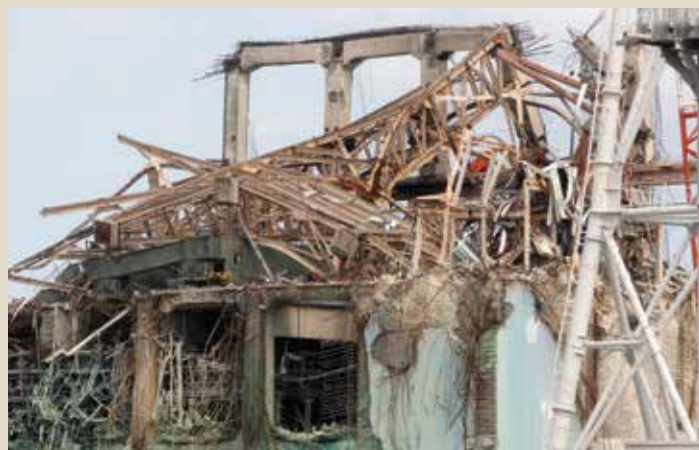
This damaged building at the Fukushima Daiichi nuclear power plant was photographed one year after the earthquake and tsunami.
