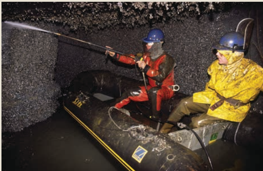
A worker uses a power washer to remove mussels from inside a water pipe.
